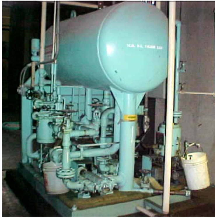
Figure 26. Seal Oil Skid
